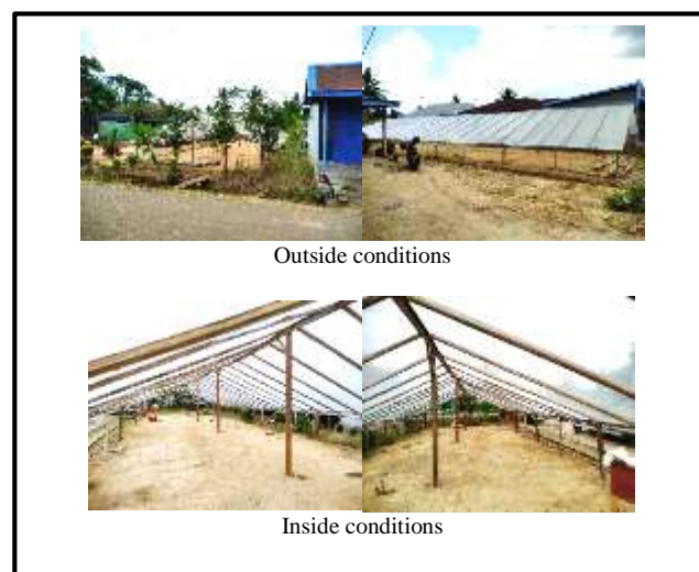
Figure 2. The condition of the outside and inside of a simple rice dryer building
