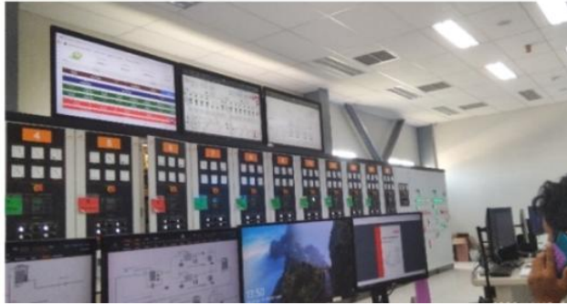
(b) Figure 1. Power Plant Location: (a) Total generating units at the site; (b) Monitoring and display system
