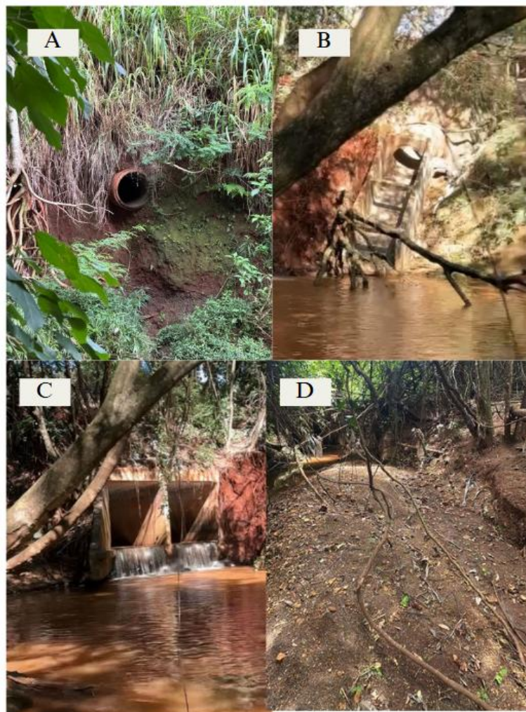
Figure 7. Drainage Structures and Siltation of Ribeirão Morangueiro
