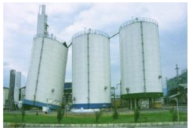
Figure 2. Damaged storage tanks (Akinci and Kilic, 2002)
