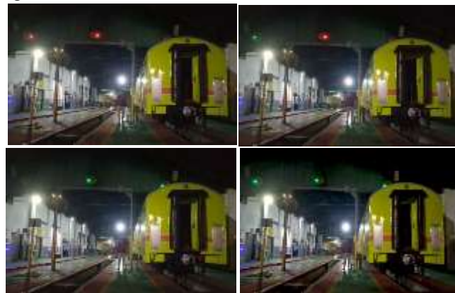
Figure 8. Functional test of solar-powered LED point signal indicators at the railway maintenance depot
