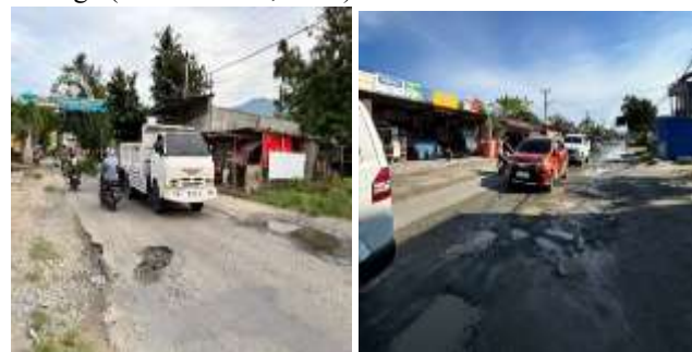
Figure 1. Pavement Deterioration on the Guru Tua Road Section
