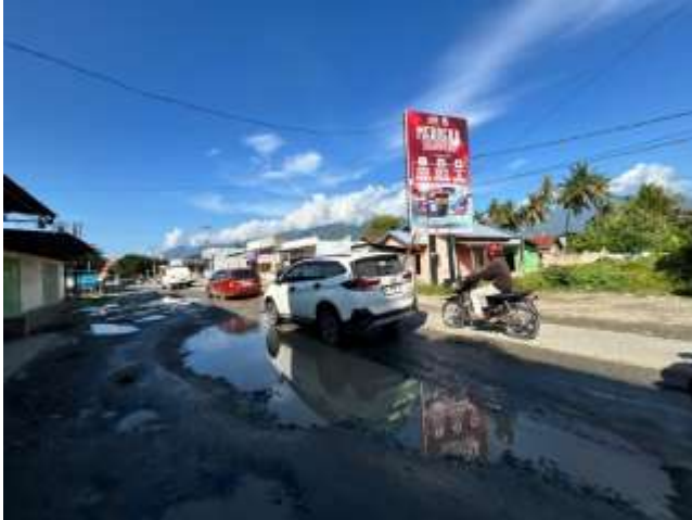
Figure 5. Severe Distress Condition at STA 02+300 – STA 02+400
