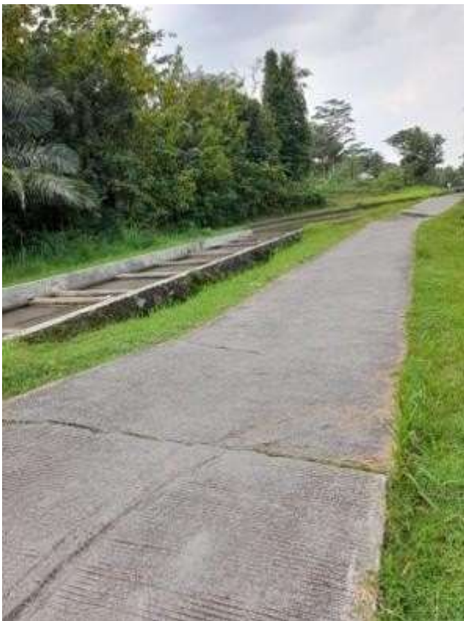
Figure 3. Shows the symptoms of landslides, which are characterized by collapsed and moved roads
