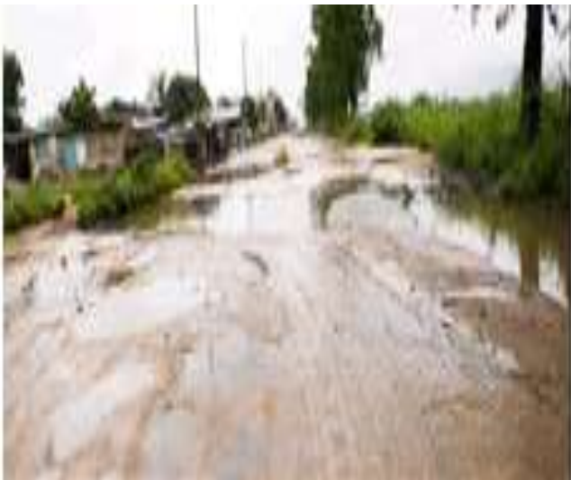
Figure No. 03: Degradation of a secondary street
