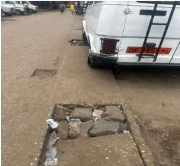
Figure No. 02: Damage on the Carrefour Adjarra Docodji - Carrefour Agata section
