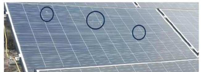
Figure 12. Condition of the solar panel surface before cleaning
