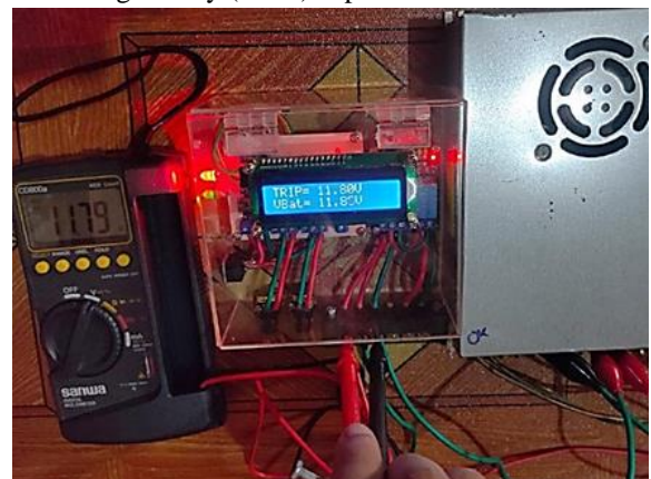
Figure 9. Low Voltage Relay Trip Execution Test
