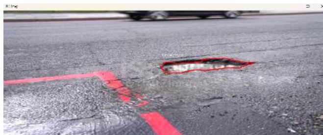
Shows that the Pothole is being detected by the model.
