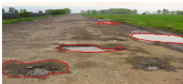
Shows that the Multiple Potholes is being detected by the model.
