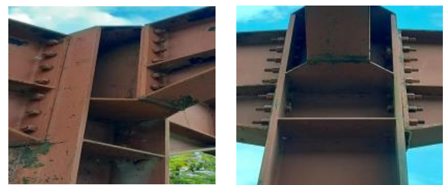
Figure 4. The condition of the bolt and weld connections is rusty
