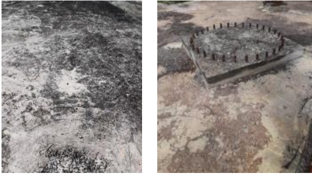
Figure 5. Condition of the floor plate and pedestal column anchors
