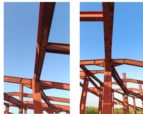
Figure 3. The condition of the columns and beams is rusty and peeling
