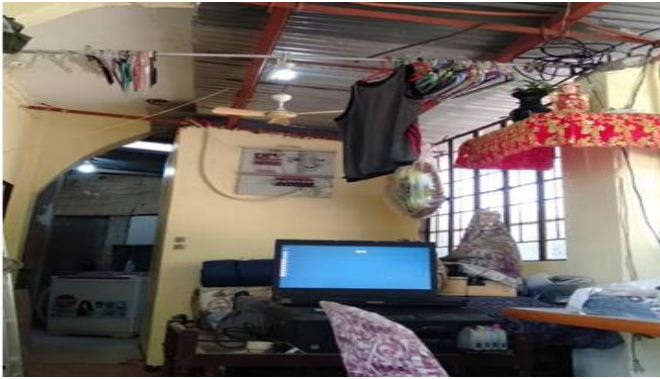
Fig. 14 Wireless Light Controller on Tailoring Shop.
