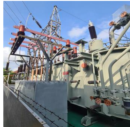
Figure 4. Transormator 1 Bungaran Substation
