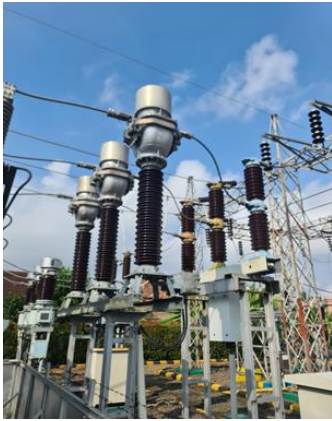
Figure 5. Lightning Arrester on Transormator 1 Bungaran Substation
