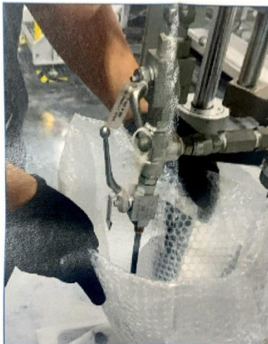
Figure 3. Process drain nozzle A
